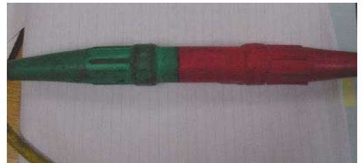
Photo No3 – "Type Two" Colour Coded Connectors, shown incorrectly interconnected
