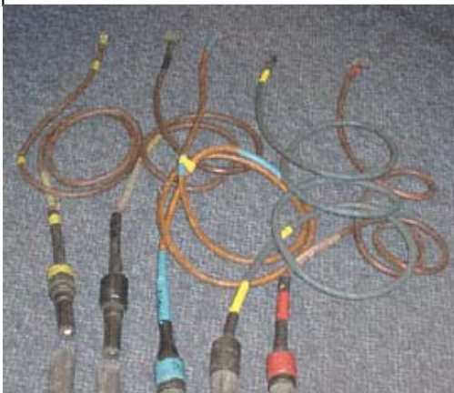
Photograph No. 7 , showing examples of ‘single core’ cables with ‘open tails’ to make the connections to a supply
