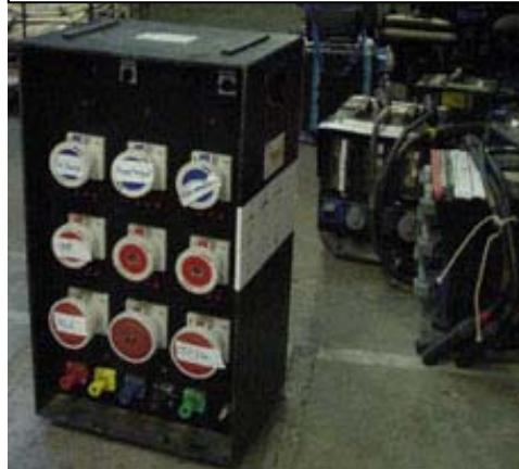
Photograph No. 8 . Showing example of Distribution Unit with ‘Ceeform’ type outlet connectors, with Type 3 inlets to old colour scheme.
